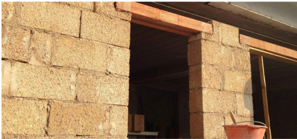
Installation of a clay lintel on a wall made of Blocco Ambiente®
