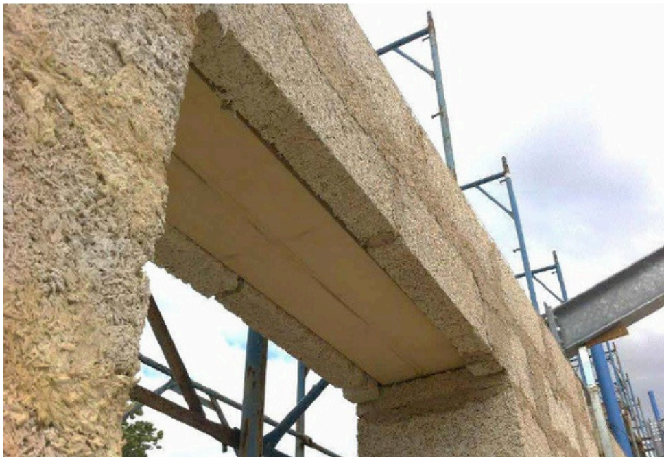
Installation of a dried wood lintel on a wall in Blocco Ambiente® including the correction for thermal bridges
