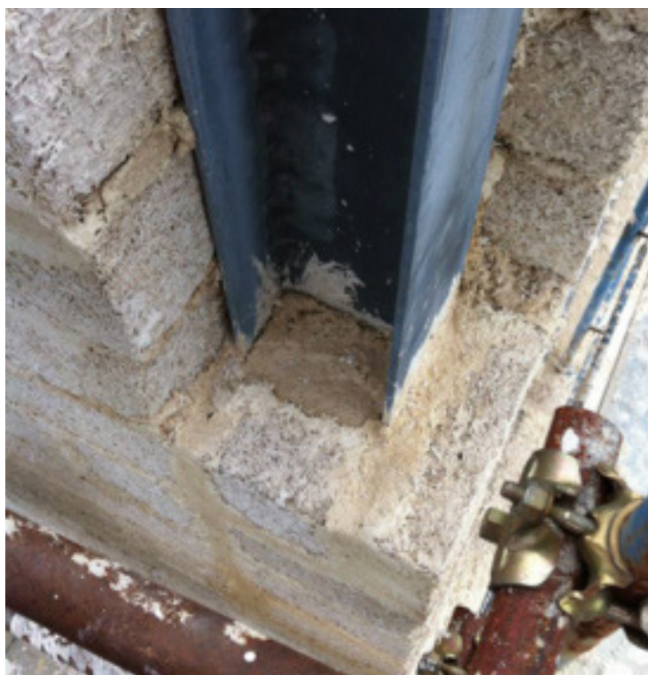
Steel frame: Thermal bridge correction with Blocco Ambiente® shaped at the corner column
