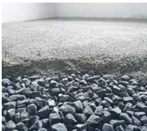
Foam glass aggregate cement-bounded, Yard Mittergroßefehn, Germany
